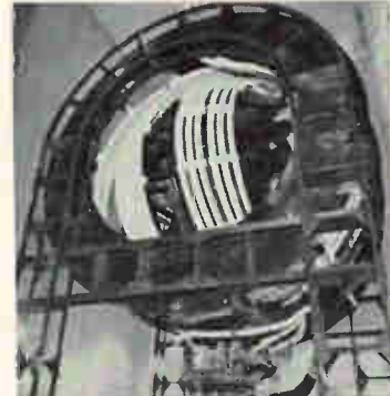
Enormous variometer coil for inductance to tune the antenna system through a range of 14 to 30 KC . . . very low frequency. These VLF radio waves penetrate the depths of the sea to submerged submarines.
