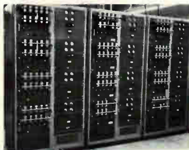
Portion of life test area, showing four-module units
