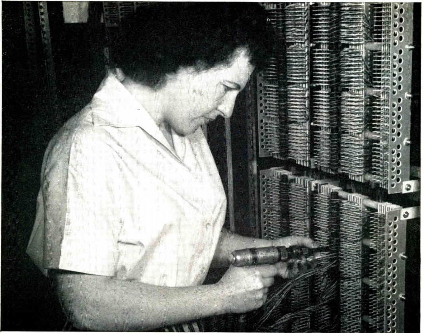
Air-powered Gardner-Denver "Wire-Wrap" tool being used by Kellogg Switchboard and Supply Company, Division of International Telephone and Telegraph Corporation.
