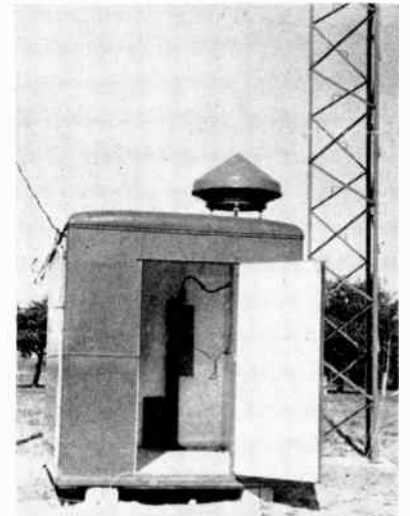
Guyed tower appears at right of one of the Raytheon radar receiver stations
