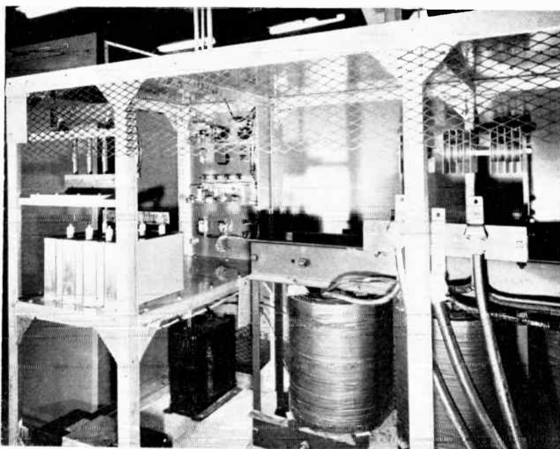
Back view of 8,000-volt, 25-amp power supply shows power transformer, thyristor assembly and filter
