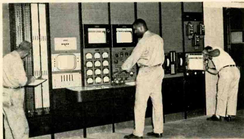
Windowless control room of Wright Air Development Center's new jet engine test stand floats on noise insulation. Technicians use tv and instruments to observe engine tests
