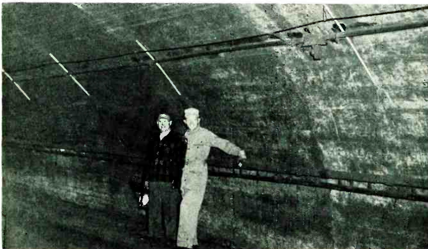
Twin-lead cable suspended in Pennsylvania Railroad Hudson River tunnel is kept as far from wall and as near passing trains as possible
