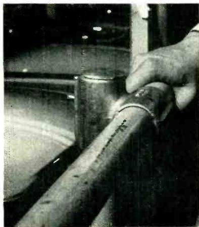
Top fitting for post of pipe fence surrounding picture tube storage area
