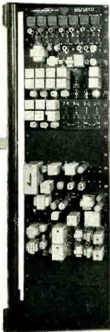
Remote Station Equipment
