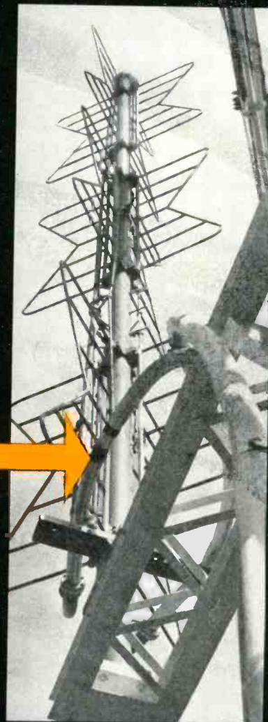
Typical TV antenna installation of Styroflex coaxial cable as a power line from station transmitter to antenna.
