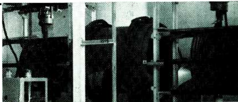
Mammoth variometer of litzendraht cable is tuning element of power-amplifier tank circuit
