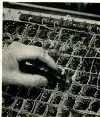
Using conical tool to spread out tube socket terminals after wiring is completed
