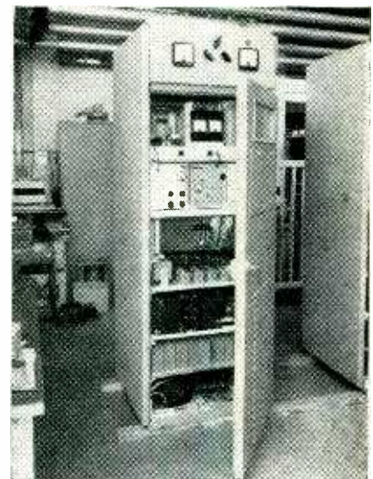
One of the 660-watt unattended transmitters. Top shelf, modulator and modulated amplifier; second shelf (left to right) submodulator, monitor unit, r-f amplifier; third shelf (top) contactor panel, (bottom) bias rectifier chassis. The lower three shelves contain the high-voltage rectifiers and auxiliary rectifiers
