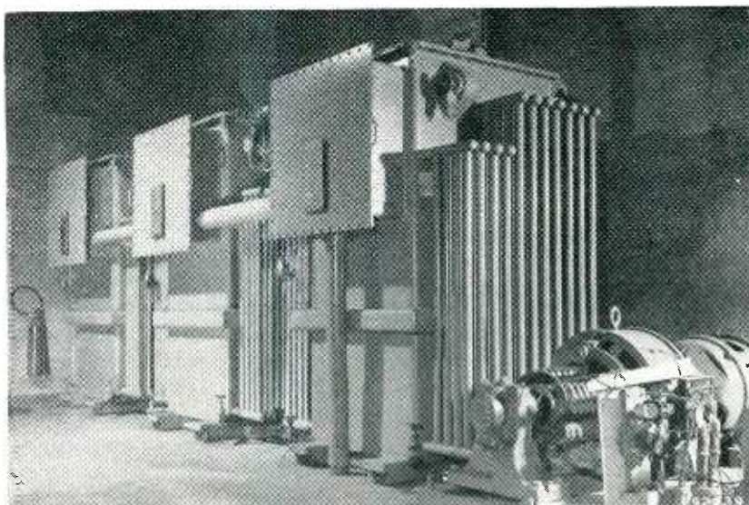
Magnetic amplifiers for controlling 1,800-kw 60-cps power supply for r-f heater on tin reflow line. Motor-generator set supplies d-c control power
