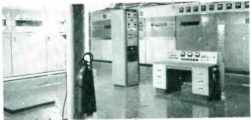
Short-wave transmitter (left) and 150-kw broadcaster (center) are located around hold. Massive hatch in deck (this side of control console) gives access to power-supply equipment in lower hold
