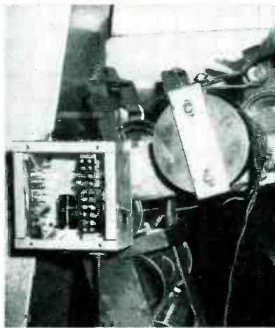
Marker installation on can run, with cover of marker circuit control box removed
