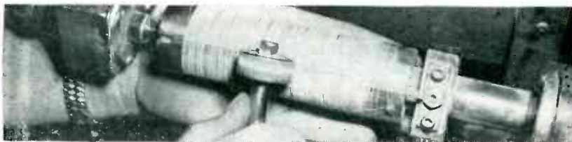
Using steel roller, resembling roller-skate wheel mounted on shaft, to crush insulation over flat cutoff anvil in mandrel
