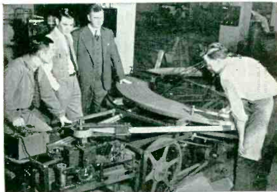
Seven miles of Revere copper bus bar were wound into great coils for the cyclotron electromagnet. The University built the winding machine itself, and wound the coils in its own shop. The special Revere bar is soft temper, free from scale, with rounded edges.
