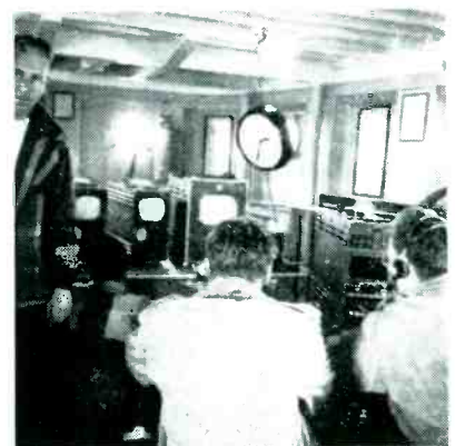
FIG. 10—Control room showing switching unit, camera control units and master monitor
