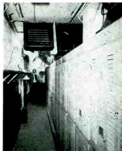
FIG. 1—Cooling radiators used to refrigerate the main amplifier room of a public address system are shown suspended from the ceiling
