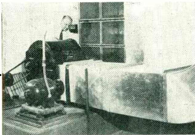
Typical blower and associated ductwork for a broadcast transmitter
