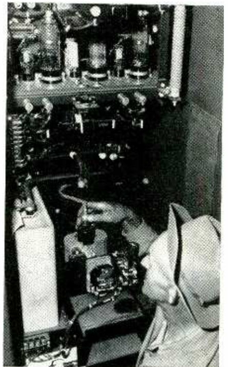
Electronic control cabinet for the fish screen
