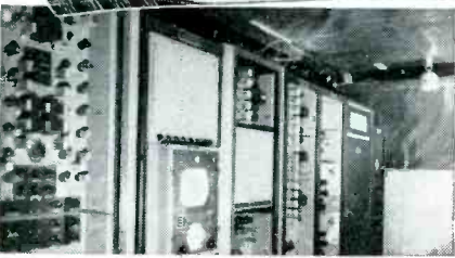
Photo courtesy of Sentinel Radio Corp., Evanston, Ill. This Central Control Room in a modern Television and Radio manufacturing plant is lined with Copper Armored Sisalkraft that eliminates stray signals and electrostatic interference.
