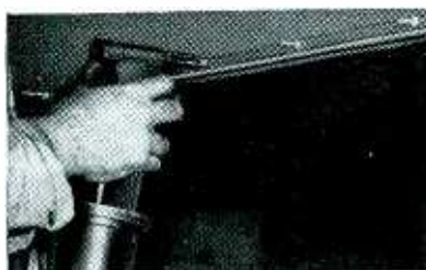
SCREWS WORK LOOSE. Cherry Rivets replace sheet metal screws in construction of refrigerated creamery trucks at Los Angeles Automotive Works. Screws had a bad record: 60% of screws would work loose within 6 months. Cherry Rivets have a perfect record of tight, vibration-resistant joints.
