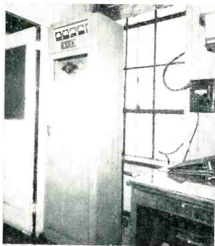
Remotely controlled f-m transmitting and receiving equipment installed in penthouse near the antenna
