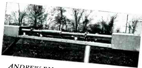
ANDREW FM-AM isolation section with cover removed, revealing two 3 1/8" FM transmission lines and expansion joints.
