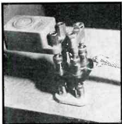
Fewest possible alterations should be made in changing connections. For series substitution, connection is arranged so that removing plug jumper at right inserts the mica capacitor in series with cable and at the same time removes the short on the cable
