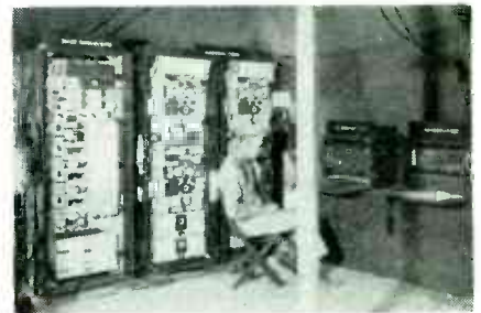
Radio relay terminal equipment as set up in the field
