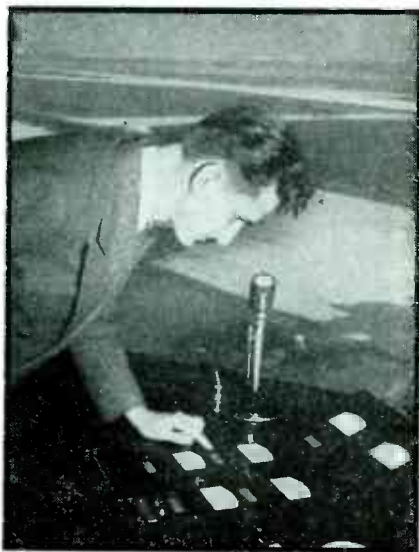
Instrument console used in control tower for operation and supervision of localizer
