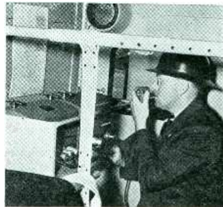
Transmitter-receiver installation in a Chicago defense corps ambulance. Map on wall shows location of city hospitals
