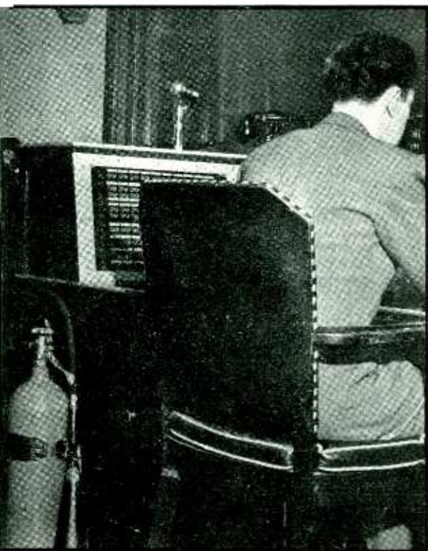
A portable carbon dioxide fire extinguisher in a studio control room at Radio City. The tank contains 15 pounds of carbon dioxide, sufficient to extinguish any fire which might start in the control panels
