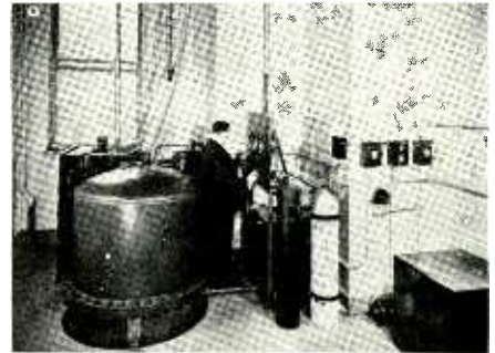
Upper portion of million-volt X-ray installation
