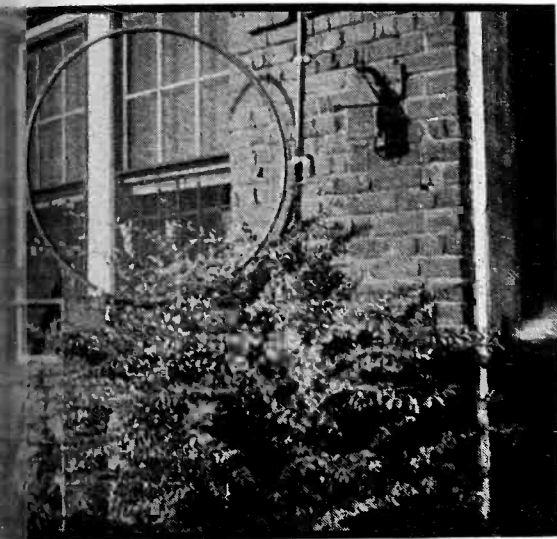
Fig. 11—A clever expansion system in use at WMPS, consisting of a loop in the line
