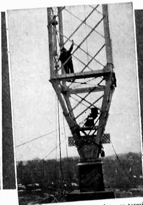
THE BOTTOM of the steel tower terminates in a point to rest on the porcelain insulator, which was wood-sheathed during erection for protection.
