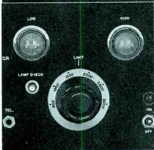
When the transmitter deviates from the assigned frequency by a predetermined amount, one of the warning lamps on the panel lights and indicates direction of deviation.
