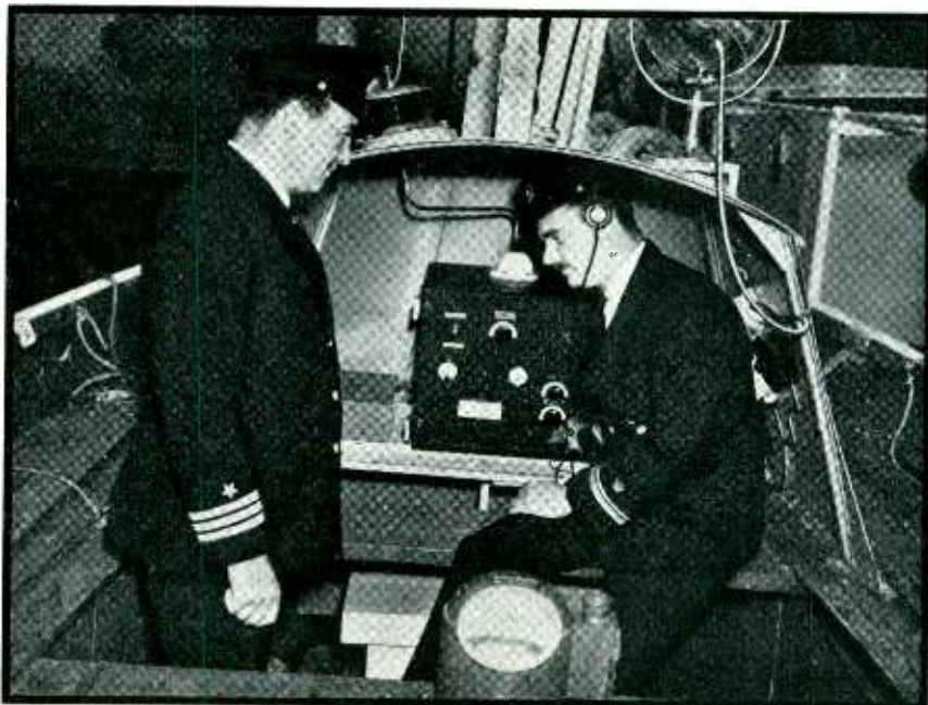
Two-way radio equipment is now compulsory on motor life-boats of all passenger liners. This typical equipment is installed on the S. S. Pennsylvania
