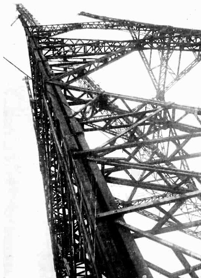
Timber-frame towers have been used extensively in Germany. Here is construction view of the new Tegel station near Berlin, to be opened this month
