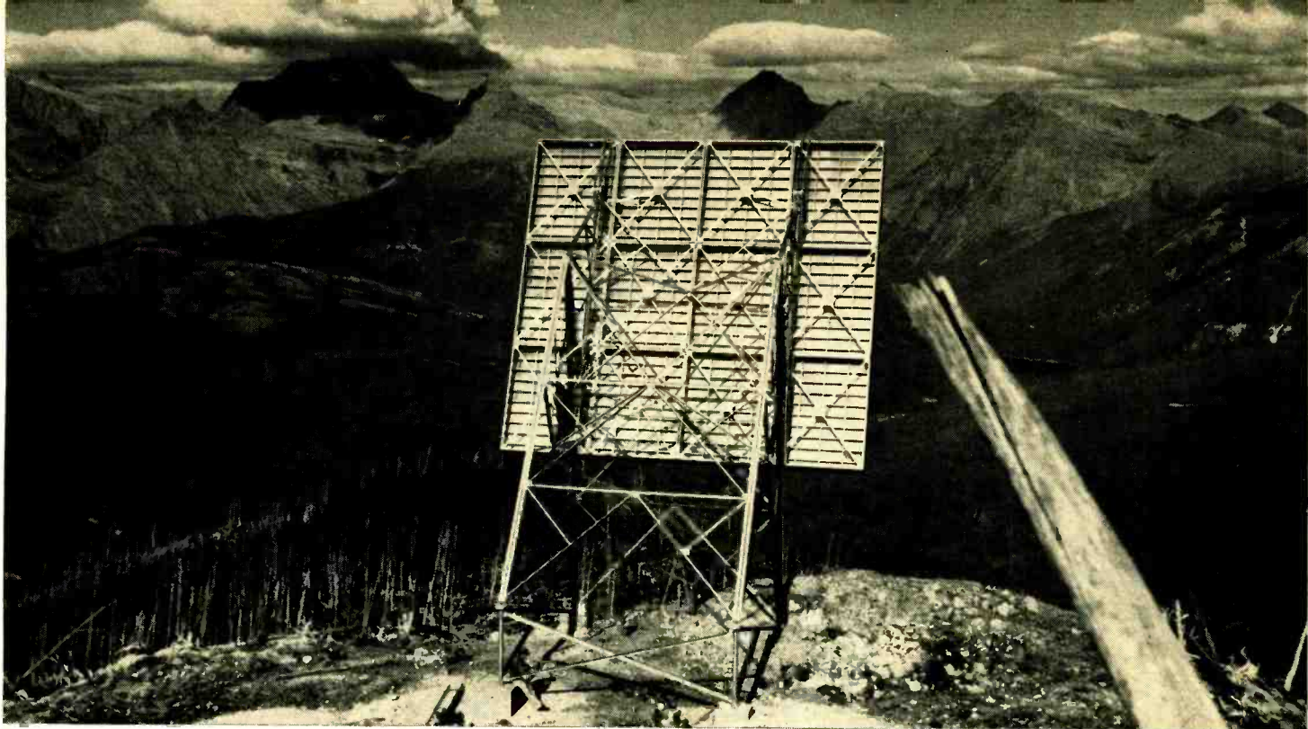
This passive repeater was installed high in the mountains of Glacier National Park, in Montana, for a large microwave radio telephone system.
