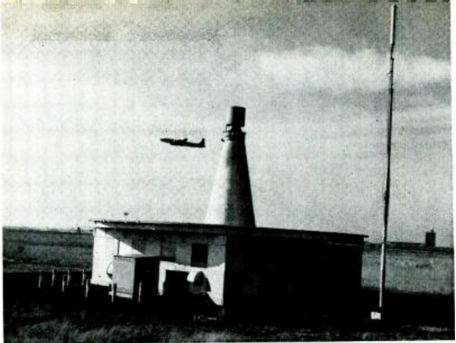
VOR and TACAN transmitter site. The main VOR antenna array is housed in the base of the cone on top of the building. It is a four-loop antenna assembly. The cylinder on top of the cone is the antenna for the Air Force-developed TACAN navigation system. The vertical antenna on the pole to the right of the main building is a distance-measuring equipment (DME) antenna. DME is currently being discontinued.
