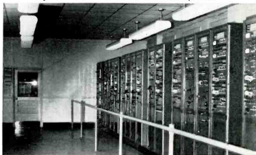
Fig. 12. View of control room of Baltimore traffic department.
