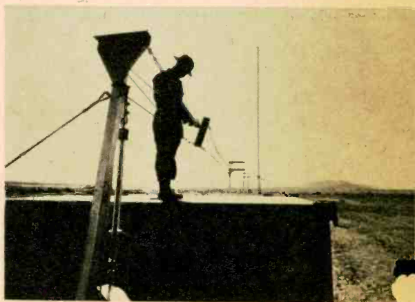
Atop transmitter shelter, GI tightens feed line carrying 50 kw to one of nine antennas included in U.S. Army's Flying Radio City, built by Gates.
