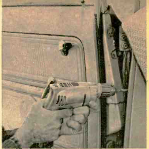
Fig. 5—If holes are not available at door edge and frame, drill a \frac{3}{8} -in. dia. hole in each for wire passage. Leave play in wire with door open.
