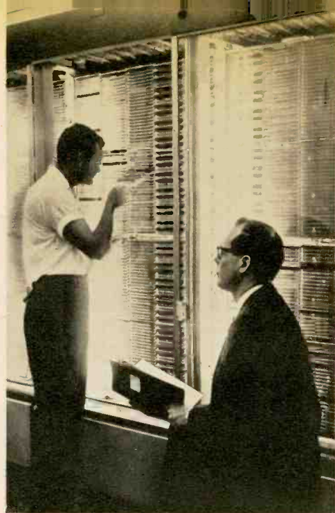
Gas tubes arrayed to form switching network. The white dots at right are tubes now in use.
