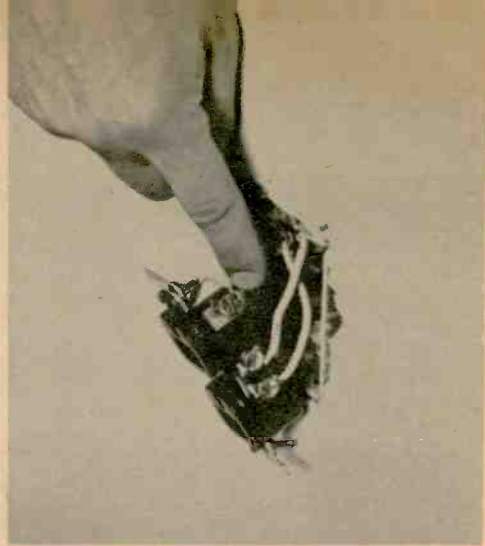
When the new 3-contact outlet is installed the third contact is grounded to the metal outlet box. Piece of braid is best for job.
