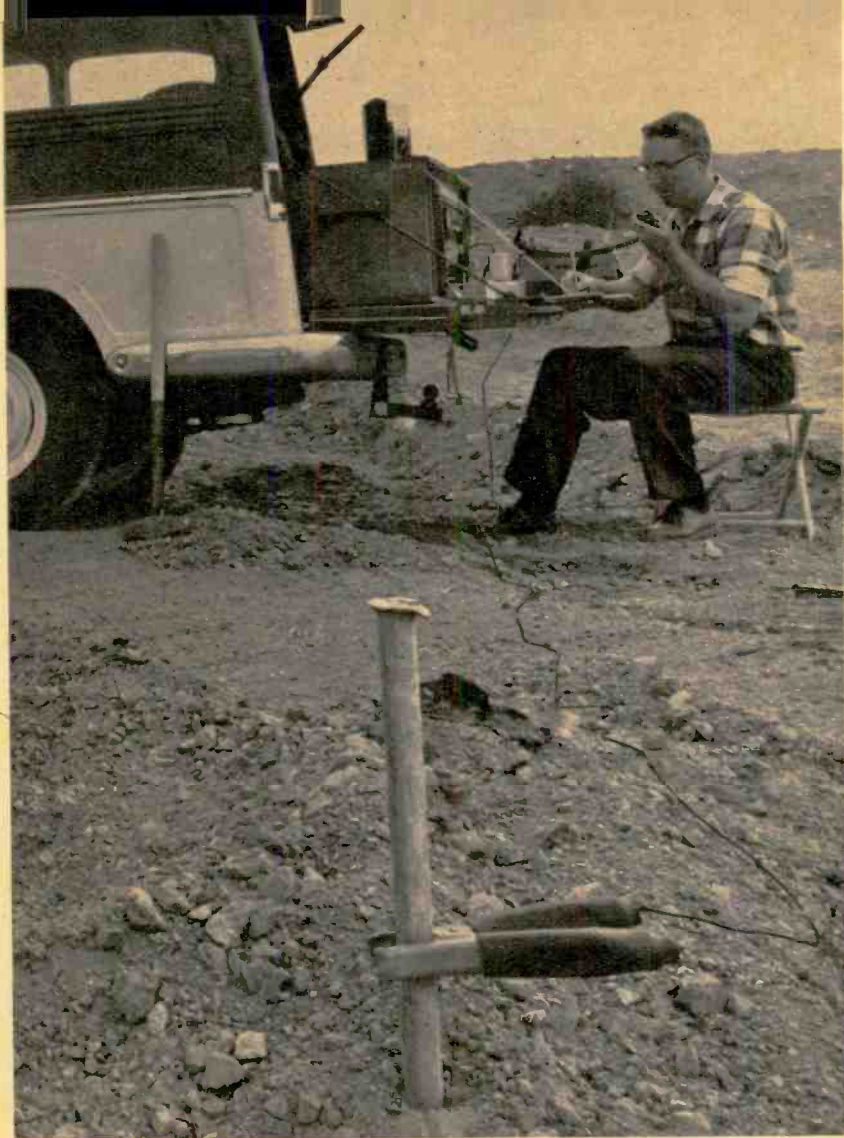
A small rig on the tailgate of a station wagon has been used by the Space Electronics Corp. for experiments with underground radio. The receiving electrode, driven in the ground with sledge hammer, is in the foreground. Note the clamped-on lead-in wire.
