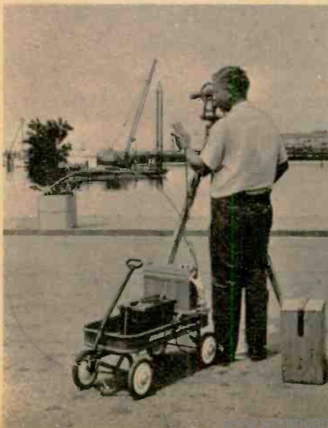
This surveyor uses what may be the world's smallest mobile radio to direct piledriver crew, talk with other surveyor across harbor.
