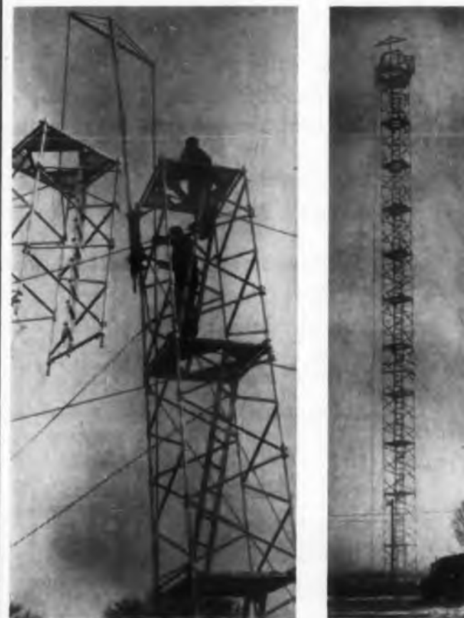
Portable aluminum antenna tower—106 ft of it—goes up in 4 hr with six men on the job, developer reports. At left, going up. Right, the full tower a few hours later.
