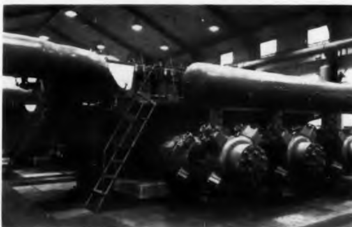
Reciprocating gas compressor station at Linden, shown with entire operating staff.
