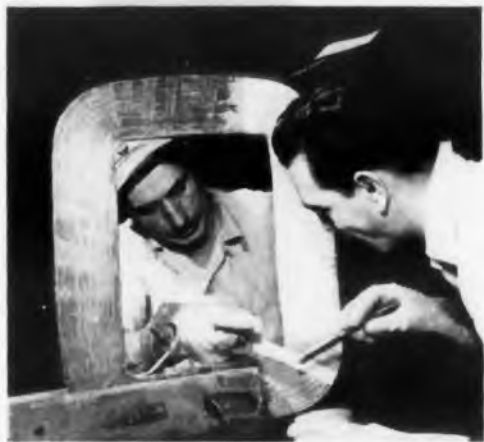
Applying Epon resin sealing compound, formulated by Epoxylite Corporation, El Monte, California, to a 400-kva transformer winding at Larsen-Hogue Electric Co., Los Angeles, Calif.
