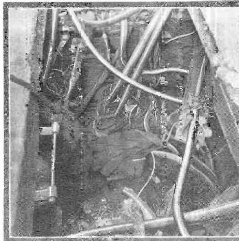
The pictures above show the tangled ruin of conduits and cables left by the April explosion.
