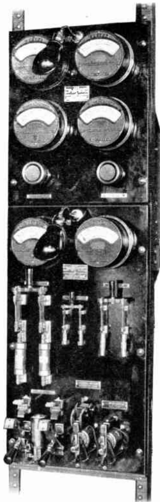
LOW-TENSION CONTROL PANEL
