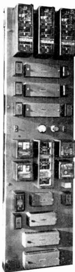
Fig. 33. Carrier-current pilot-relay equipment with distance and ground-fault backup protection, showing complete equipment for one line end
