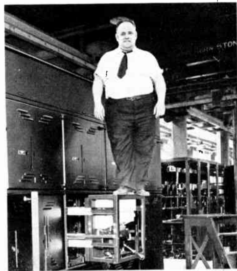
Fig. 26. Low-voltage switchboard, with sturdy, drawout air-circuit-breaker units
