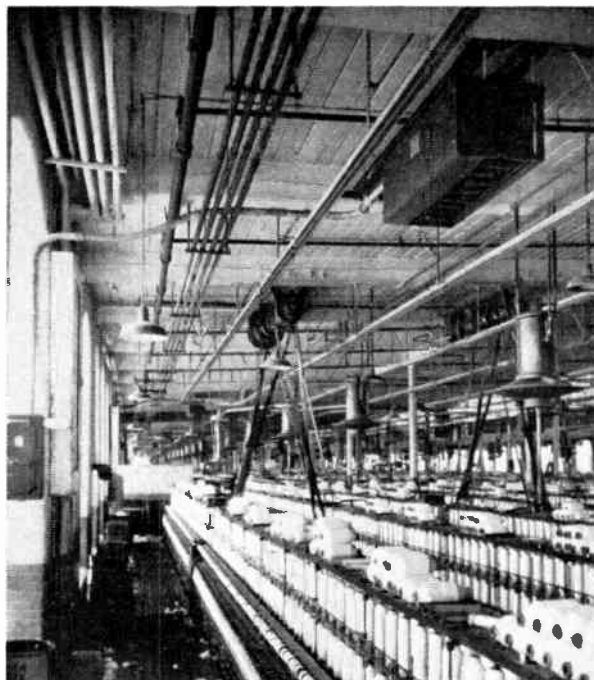
Fig. 107. Typical installation of Pyranol capacitor equipment in textile mill
