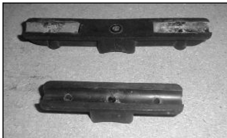
Fig 2: Another view of the element insulators. The top insulator is banana shaped due to UV exposure.
