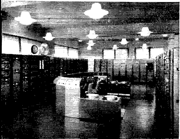
Fig. 5—The main receiving room at Ueberacker—a true ham's paradise. The 26 dual and triple diversity receiving channels use SP-600, 51-J, and AR-88 receivers working into Pioneer and Crosby single-sideband adapters and combiners.
