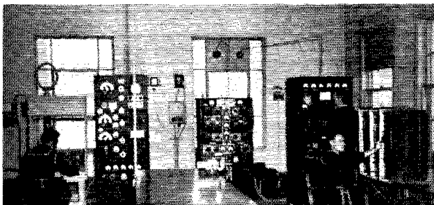
Transmitter room at the Naval Reserve Training Center, Michigan City, Indiana. The TBW transmitter at the extreme right is easily transported, with its own emergency power, and is kept in readiness to meet disaster relief needs.
