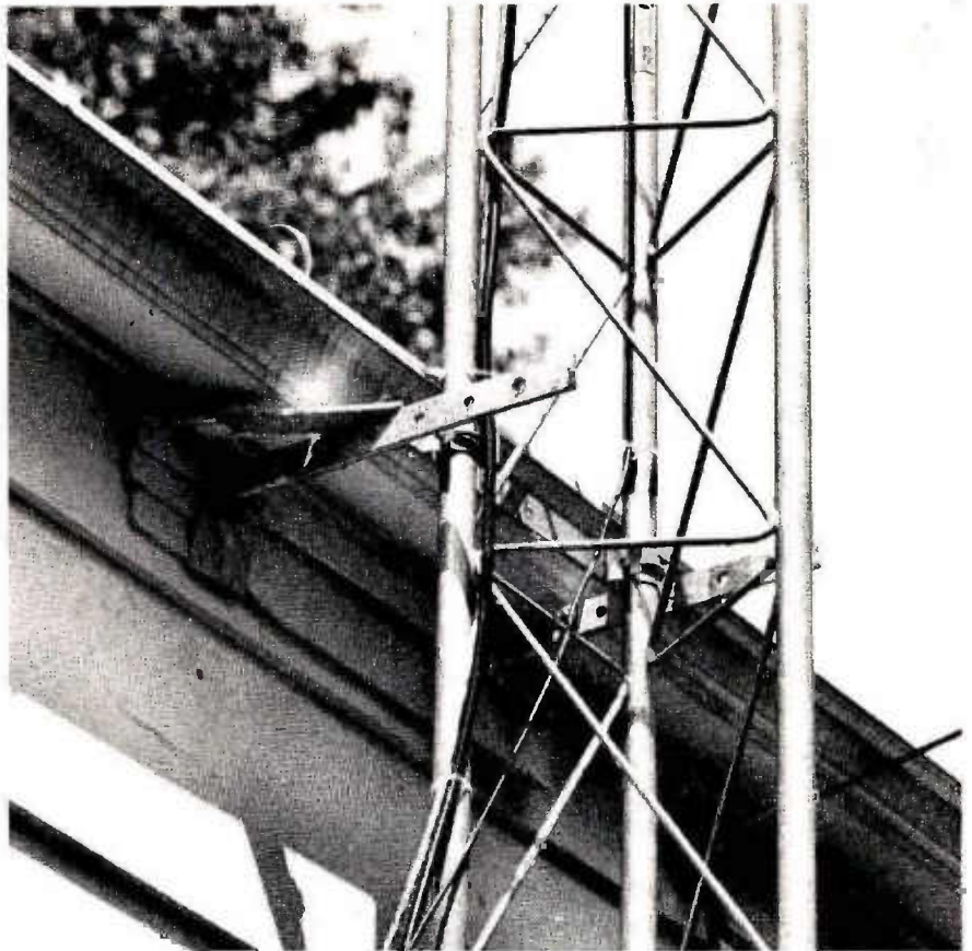
A bracket to hold the tower to the house will take the place of guy wires — up to a modest height, at least. The brackets are adjustable, but some wood shims were needed to be sure the tower was exactly plumb.
