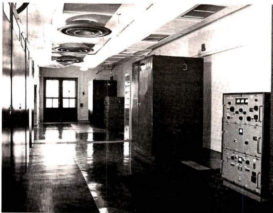
Transmitters line both sides of the corridor. The small units on the right are standby transmitters, which have been replaced by higher-powered ones. An automatic monitoring and switching system is used to change to a standby transmitter in case of failure, and to sound an alarm to bring an operator to fix the trouble ( photo courtesy Canadian National Research Council ).
