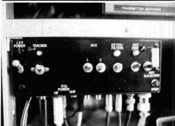
DC control panel, column of LEDs and "Stop" LED used for elevation indication on right side.
