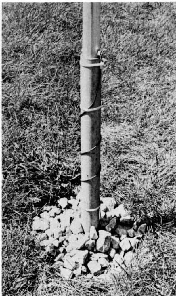
One of the ground mounts for the parasitic elements. The wire wound around the mount is soldered to three radials under the ground; it is attached to the base of the parasitic element with a wing nut.
