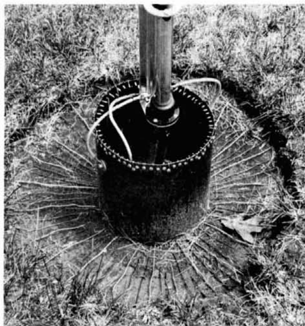
Base of the driven element showing the length of large diameter copper pipe used for terminating the radials. Narrow slits were cut in the lawn to place 72 radials around the base of the antenna.
